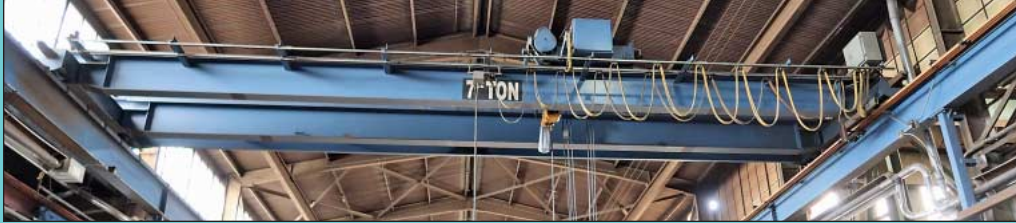
(2) 7.5-Ton x 42' Approx. Wazee Double Girder Top Running Overhead Bridge Cranes
