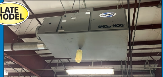
(2) UAS Smog Hog Fume Collectors
