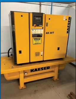
Kaeser Air Compressor
