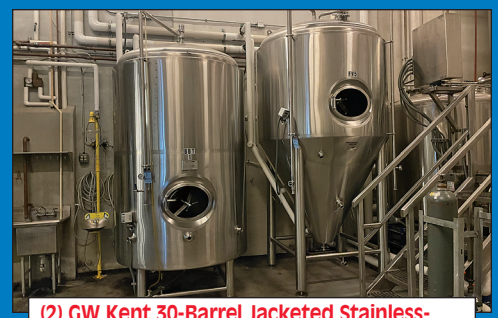
(2) GW Kent 30-Barrel Jacketed Stainless-Steel Tanks
