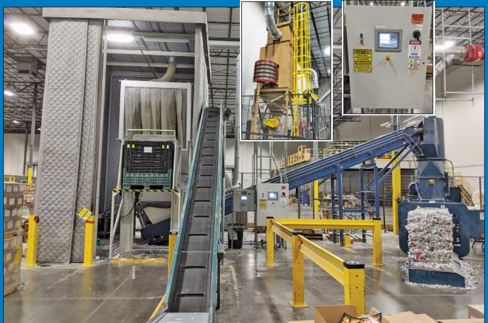
Overall View Vecoplan Shredder and Balemaster System
