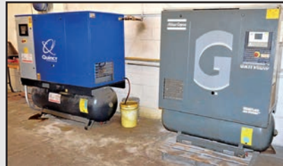
View of Air Compressors
