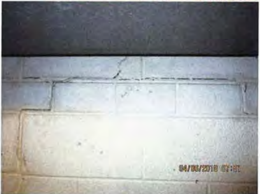
New movement of left garage wall.
