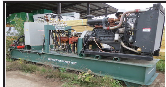
Power Unit Iveco Diesel 5,200 Hours, Low Oil Shutdown on Hydraulic Units and Motor Hydraulic Tank
