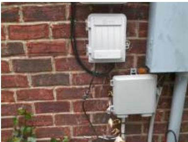
Cable Television, Telephone Grounding Wire Verified: Yes - The cable television and/or the telephone service lines appeared to be grounded.
