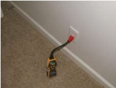
Bedroom #2: Functional - The outlets tested in this room were correctly wired and grounded.
