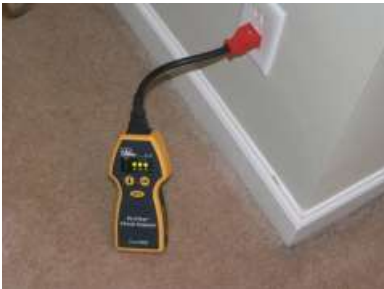
Bedroom #3: Functional - The outlets tested in this room were correctly wired and grounded.
