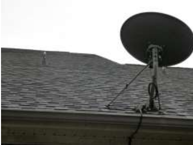
Telephone Service: Underground.
