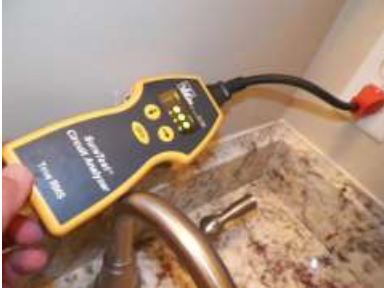
Master Bedroom: Functional - The outlets tested in this room were correctly wired and grounded.
