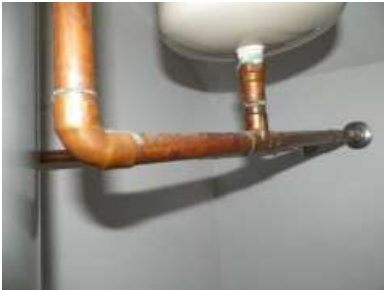
Interior Supply Piping Size: The interior water supply piping is 3/4" in diameter. It then reduces to 1/2" or 3/8" risers.
