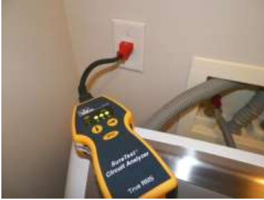
Master Bathroom: Also protected by GFCI.
